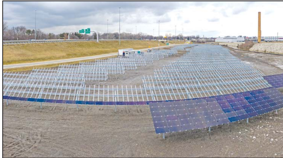
The Overland solar site, between Interstate 75 and the Ottawa River. Photo courtesy of GEM Energy
